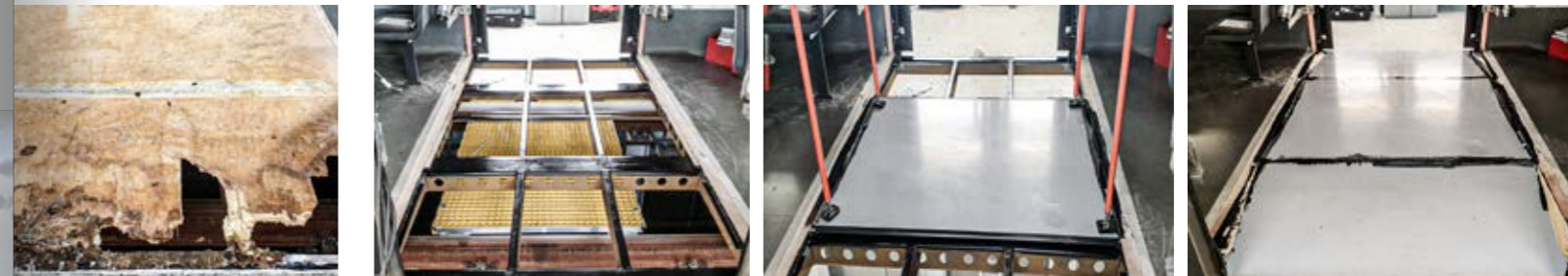
Complete Flooring Renovation: From Damaged Wood Flooring to a System of GRP Sandwich Panels
